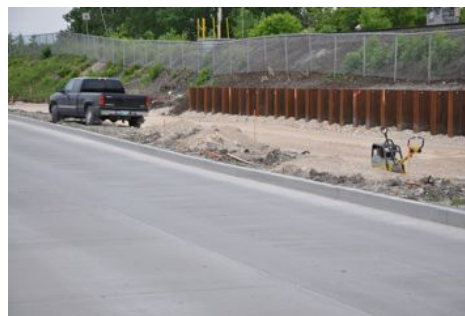
The northern end of the busway, where the southbound lane leaves Main St. At this point the northbound lane leaves the busway and crosses Stradbroke, to the left.
