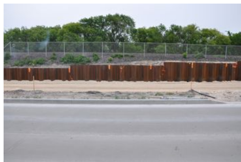
Showing the method of shoring up the embankment of the CN mainline.
