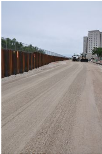
Work on the portion of the line as it curves to the left beside Donald St.
